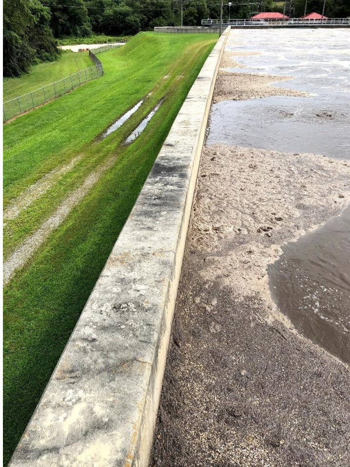
Figure 5.99 – Wheel Tracks North of Aeration Basin #2
