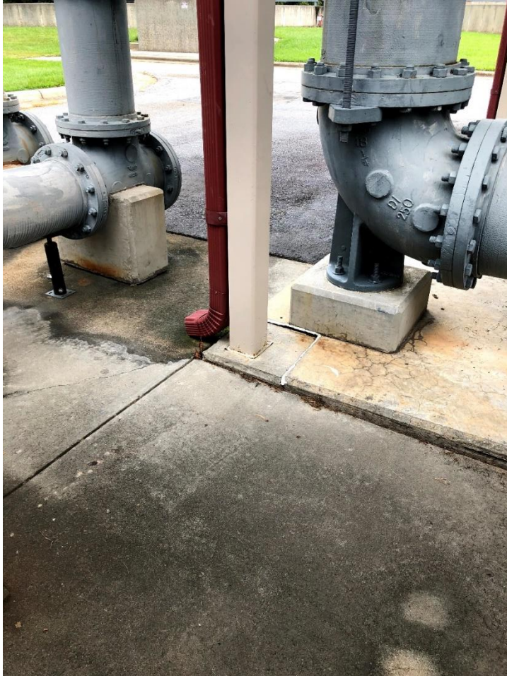
Figure 5.58 – Blower Building Column Footing Settling
