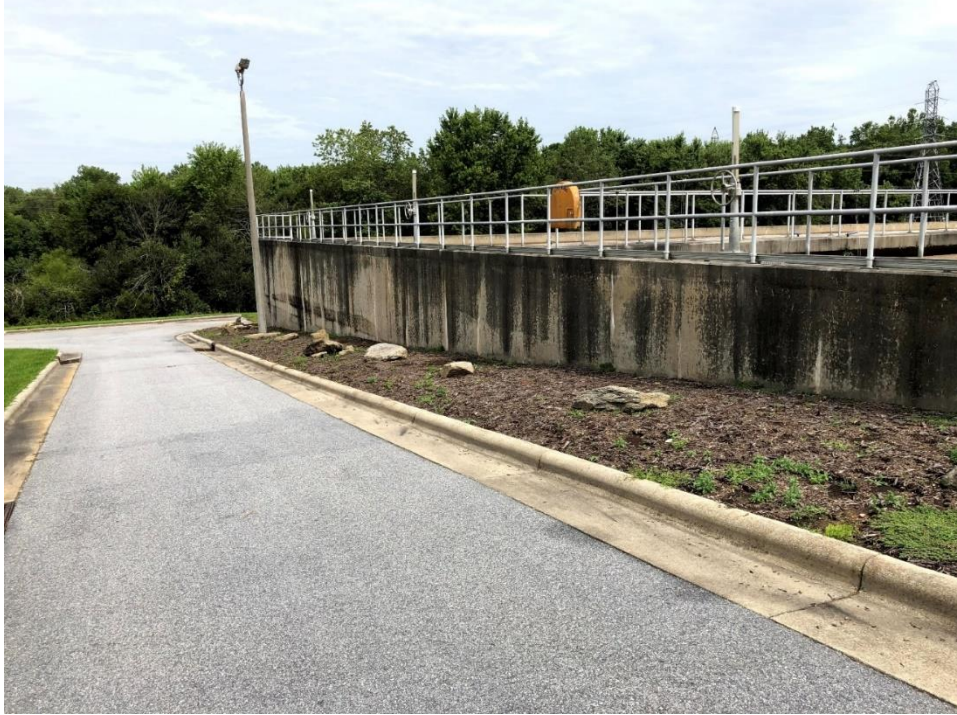
Figure 5.44 – Aeration Basins Crack Patterns on West Wall
