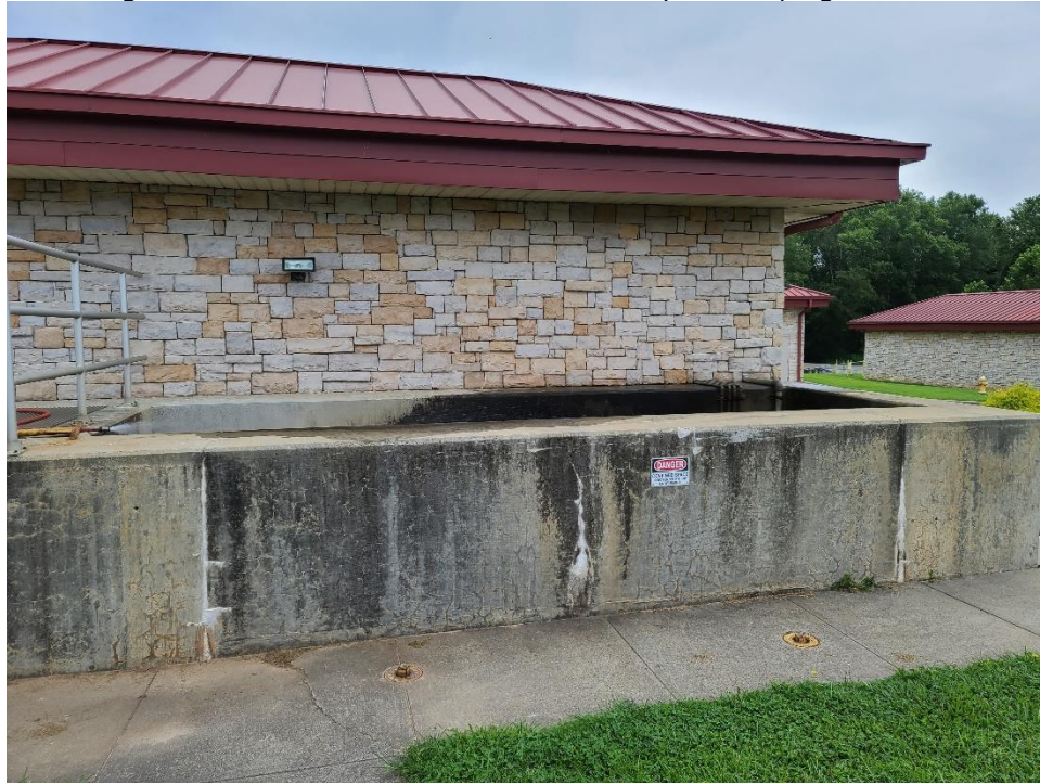
Figure 5.100 – Sidewalk Settlement at Recycle Pumping Station
