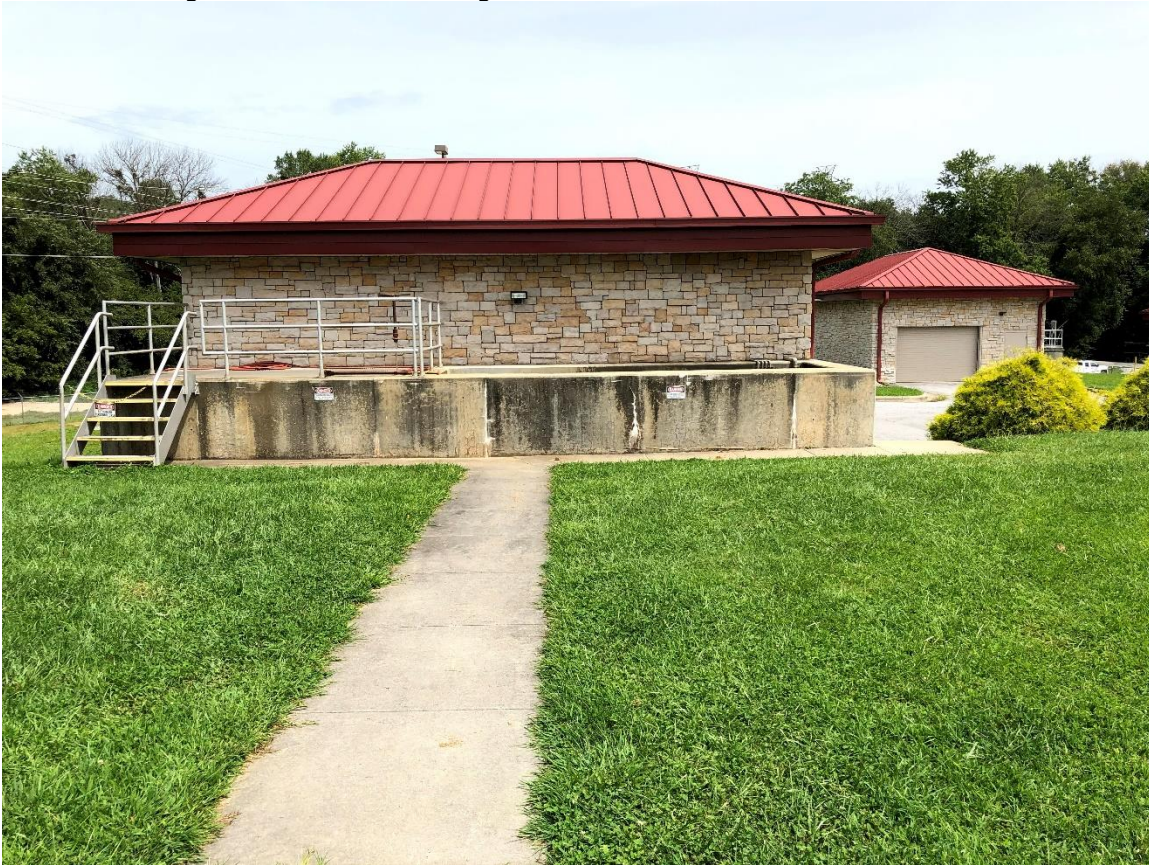
Figure 5.63 – Return Sludge Wet Well Vertical Cracks on West Wall
