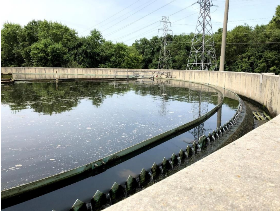
Figure 5.60 – Secondary Clarifier Effluent Weir and Launder
