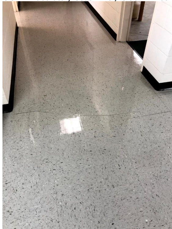
Figure 5.4 – Laboratory South Entry Crack in Floor Tiles
