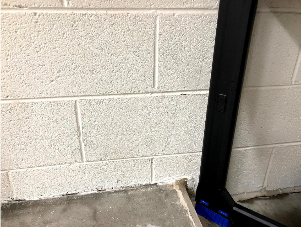
Figure 5.77 – Utility Building Hairline Cracks in South CMU Wall
