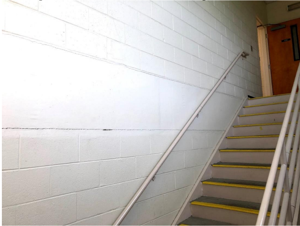
Figure 5.15 – Stairwell Horizontal Crack Along Concrete Beam
