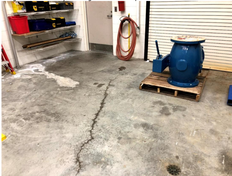
Figure 5.76 – Utility Building Linear and Map Crack Patterns on Floor Slab
