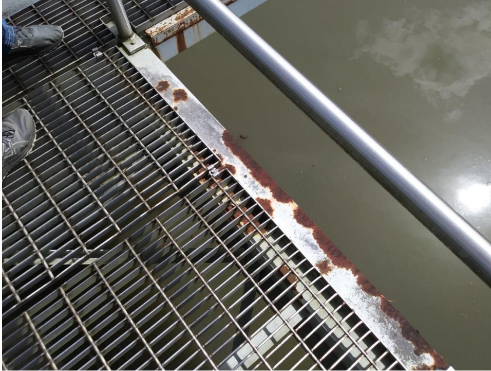
Figure 5.89 – Gravity Thickeners Rust on Top Center Walkway Framing
