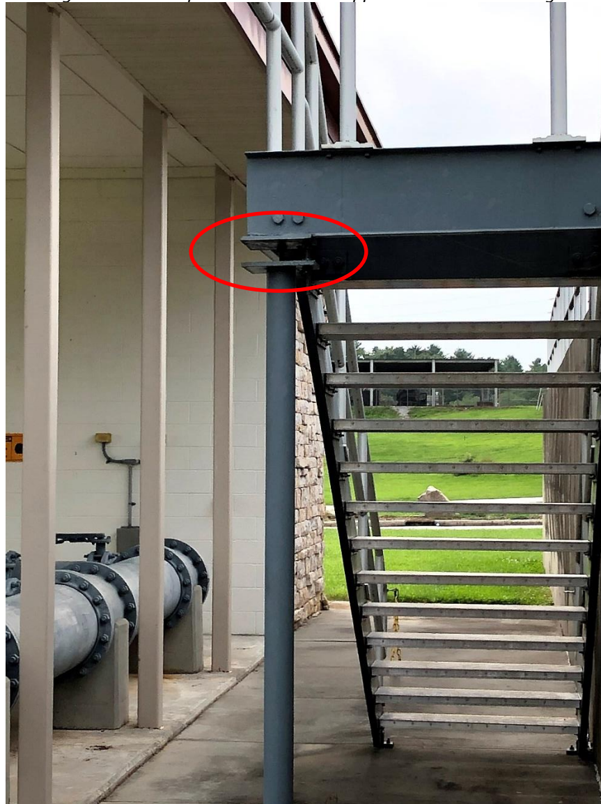
Figure 5.57 – Separation of Stair Support at Blower Building
