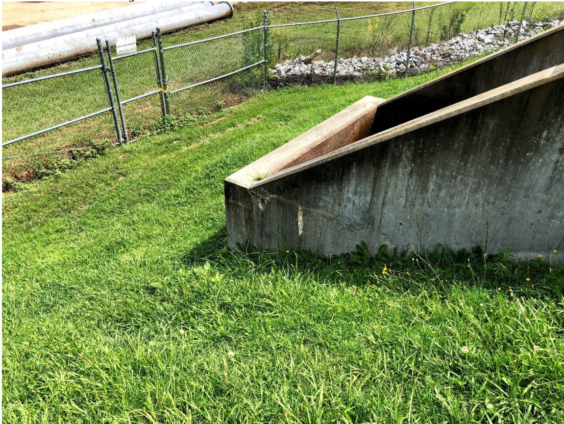
Figure 5.80 – Cascade Reaeration Cracks in North Wall
