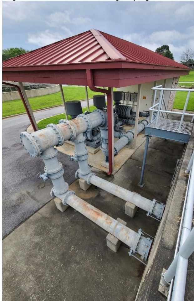
Figure 5.53 – Blower Discharge Piping Condition
