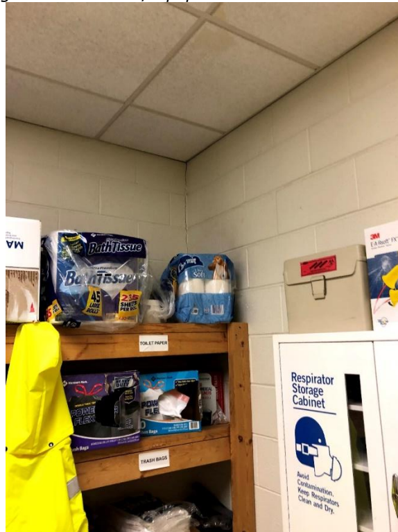
Figure 5.16 – Coat/Equipment Room Vertical Crack
