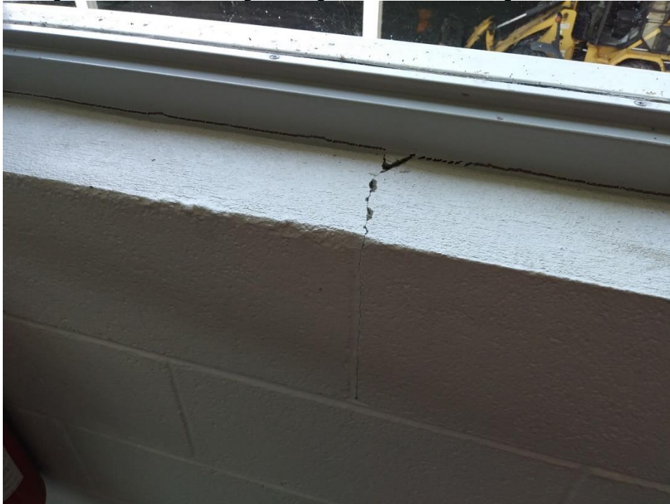
Figure 5.93 – Dewatering Building Control Room Through Block Crack
