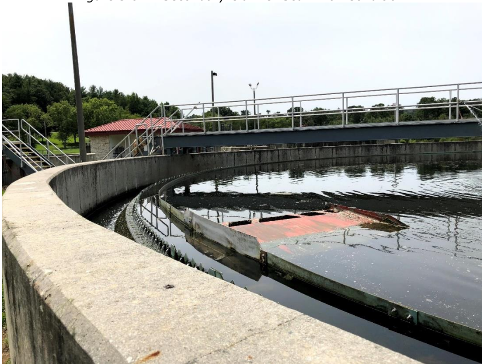
Figure 5.61 – Secondary Clarifier Scum Box Condition
