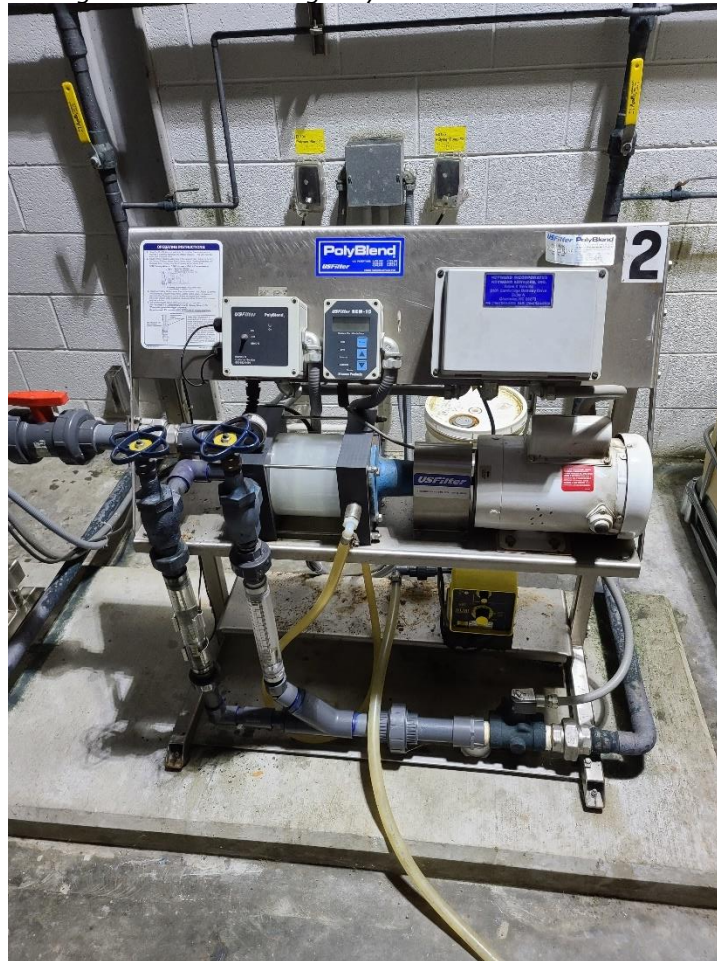
Figure 5.91 – Existing Polymer Makedown Skid #2
