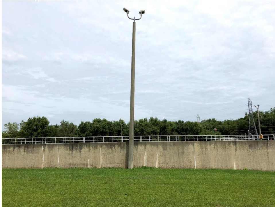
Figure 5.43 – Aeration Basin #1 Vertical Cracks on South Wall
