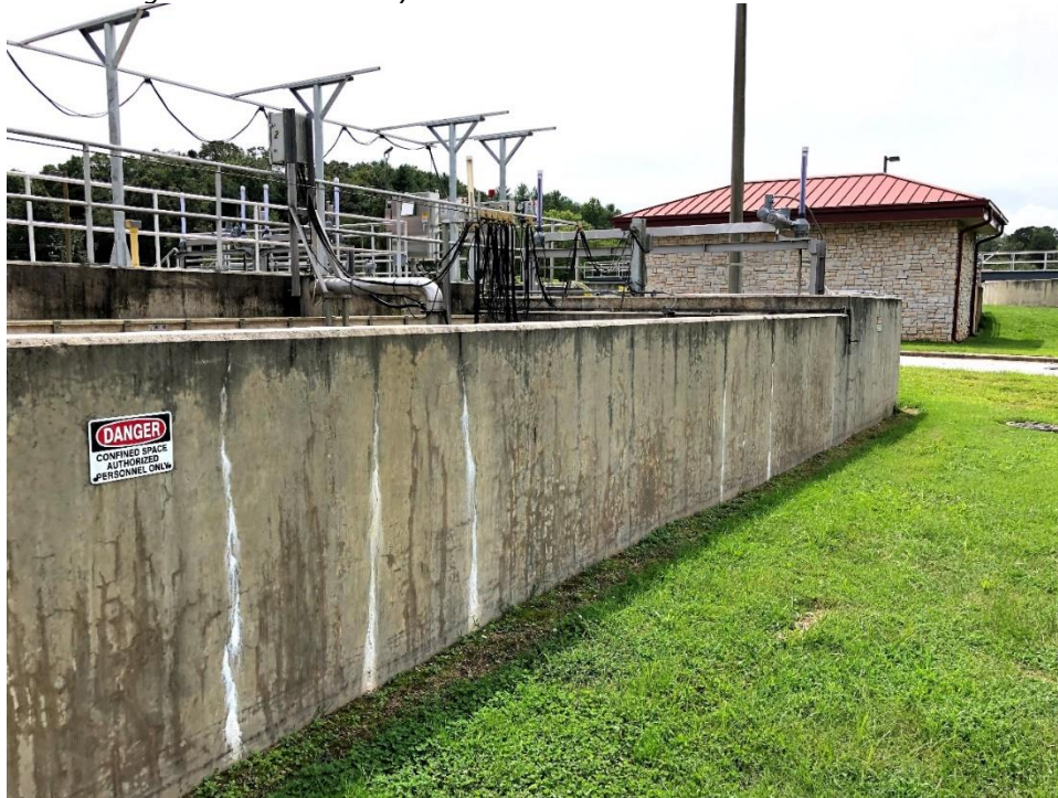
Figure 5.71 – Tertiary Filter #2 Vertical Cracks on North Wall
