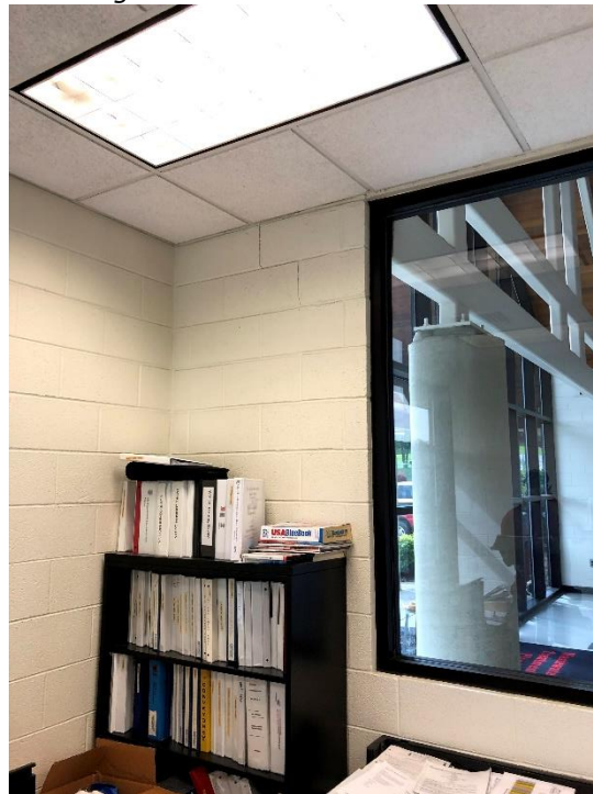
Figure 5.8 – Program Coordinator Room Cracks in CMU Wall
