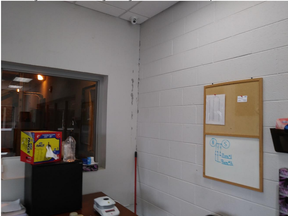
Figure 5.92 – Dewatering Building Control Room Vertical Separation Cracks
