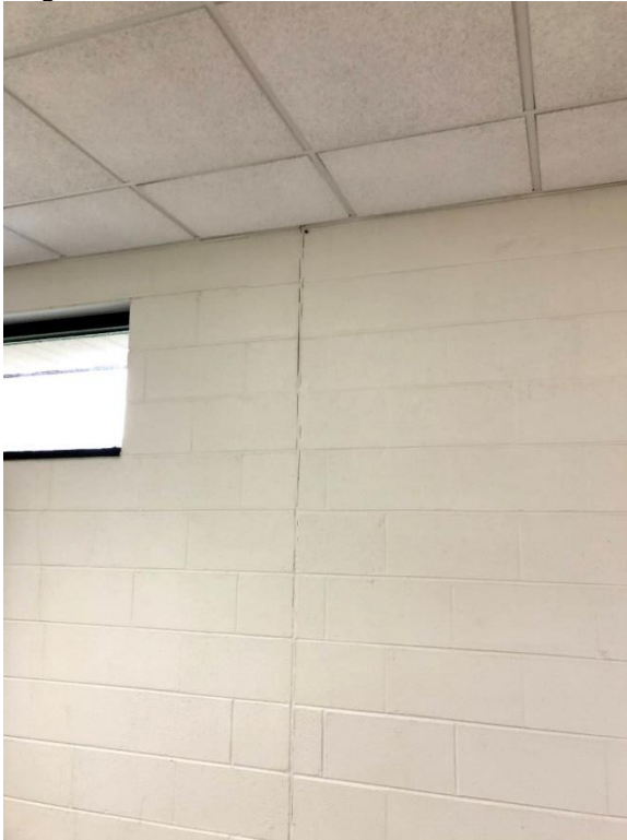
Figure 5.19 – Women’s Room Vertical Crack
