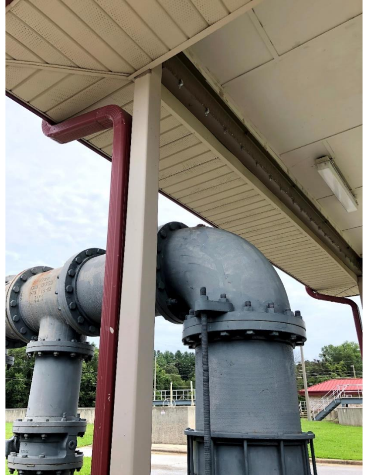
Figure 5.59 – Blower Building Column Settling
