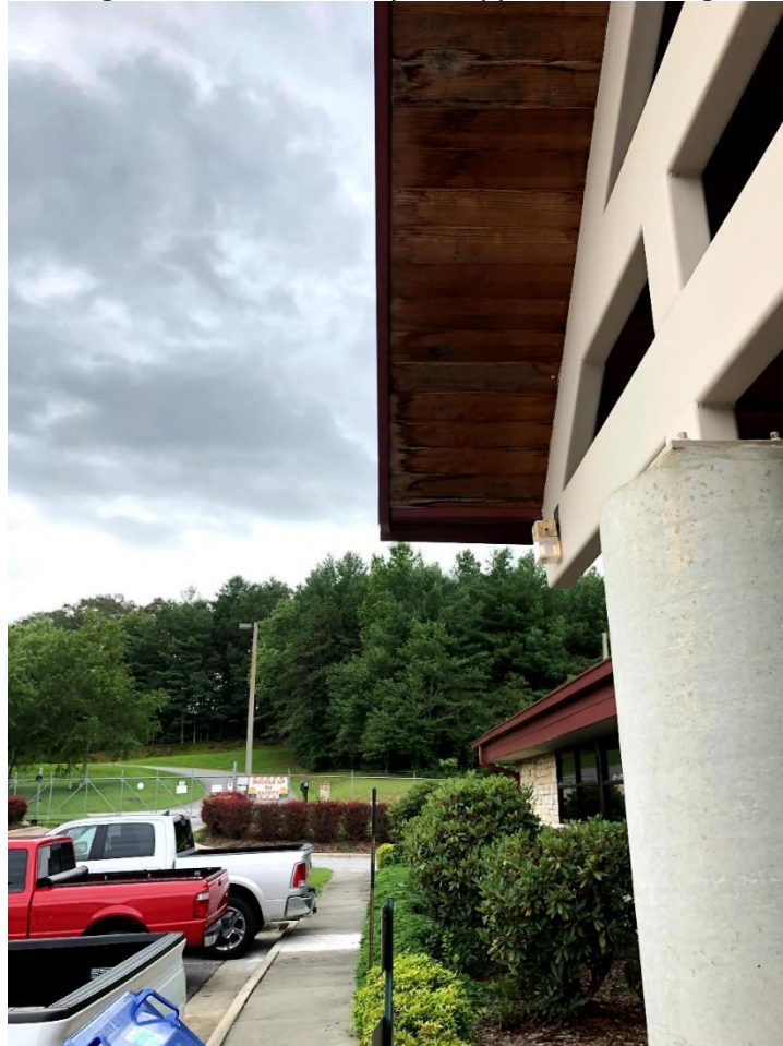
Figure 5.25 – Main Entry Canopy Water Staining
