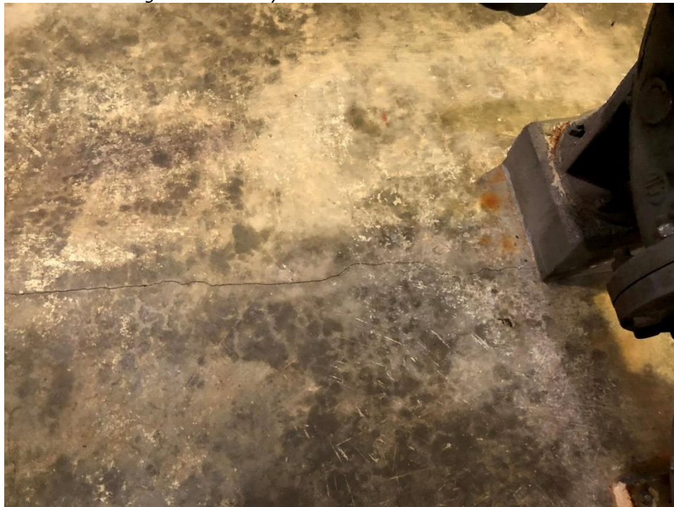
Figure 5.33 – Dry Pit Hairline Crack in Floor Slab
