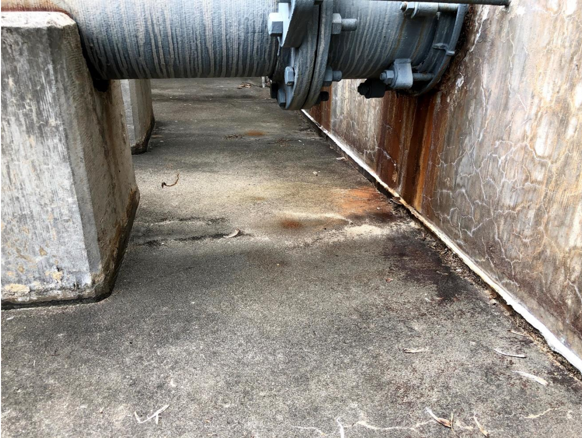
Figure 5.54 – Differential Settling of Slab-on-Grade at Aeration Header Wall Penetration
