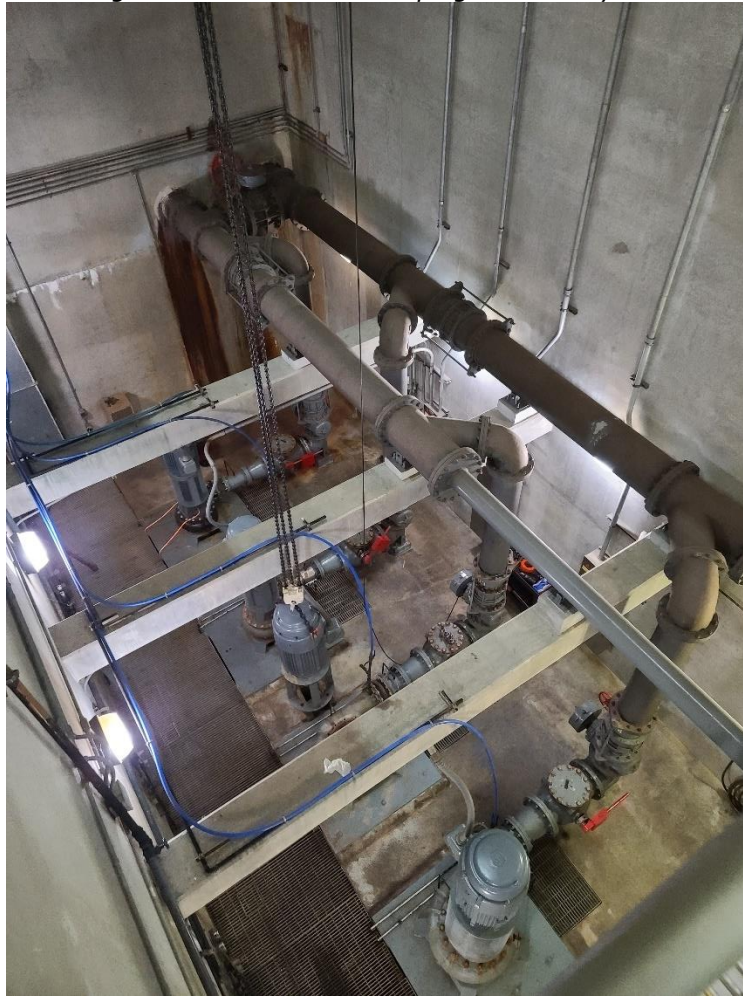
Figure 5.26 – Influent Pumping Station Dry Pit
