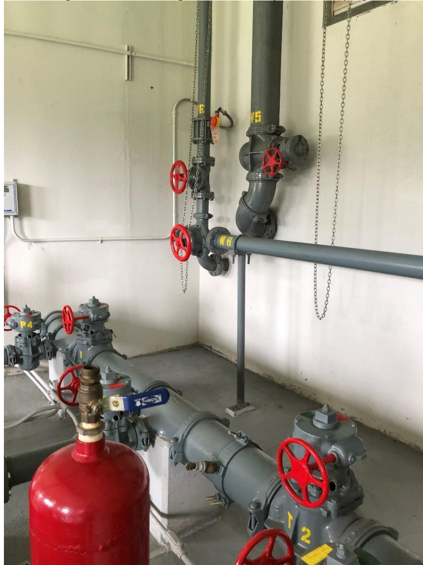
Figure 5.84 – Existing BFP Feed Pump Suction Piping
