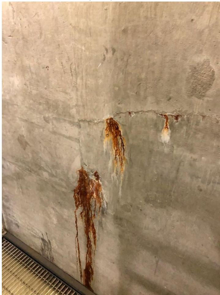
Figure 5.28 – Dry Pit Vertical and Horizontal Cracks in CIP Wall
