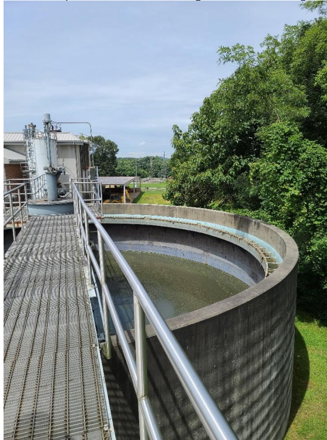
Figure 5.83 – Gravity Thickener #2 During Thickened Sludge Withdrawal
