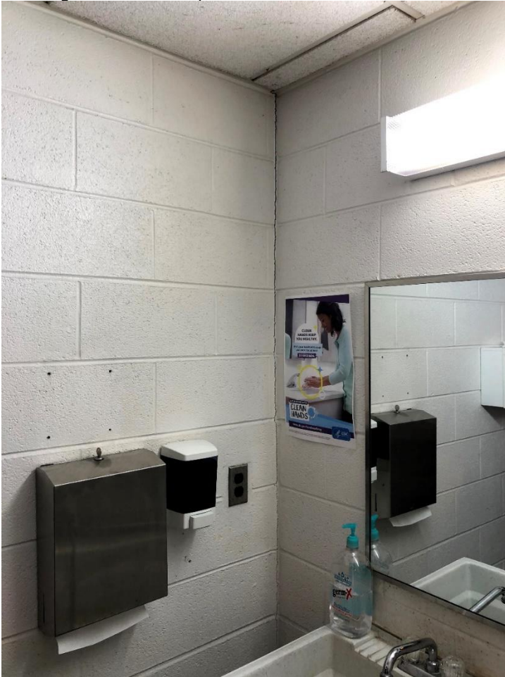
Figure 5.13 – Shop Restroom Vertical Crack
