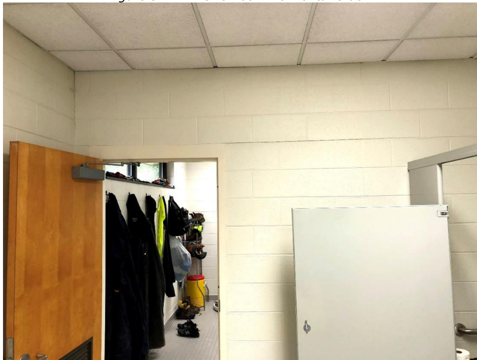
Figure 5.21 – Men’s Room Horizontal Crack
