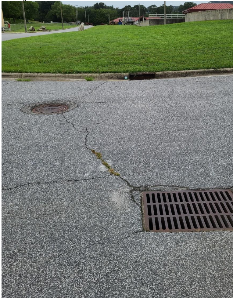
Figure 5.101 – Potential Settlement of Sewer Manhole
