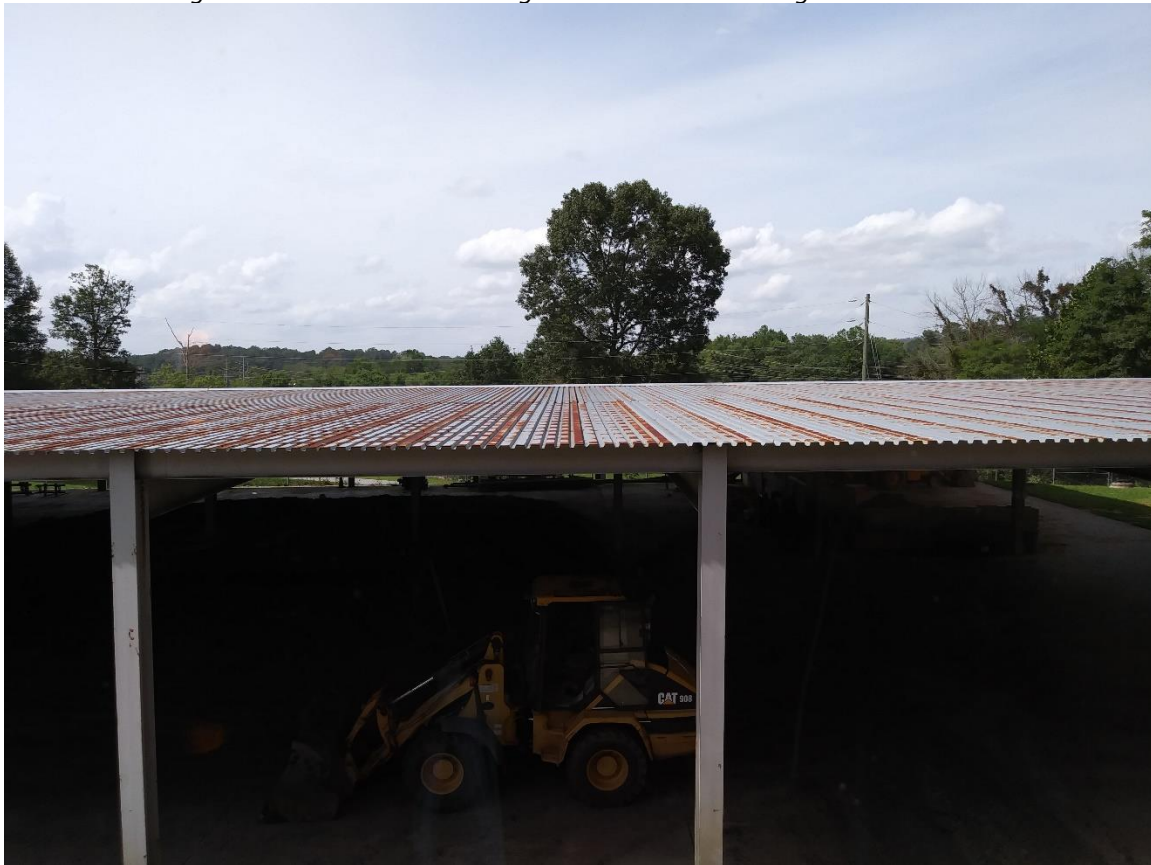
Figure 5.96 – Biosolids Storage Shelter Roof Decking Deterioration
