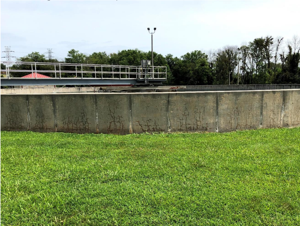
Figure 5.62 – Secondary Clarifiers Vertical Cracks Around Perimeter
