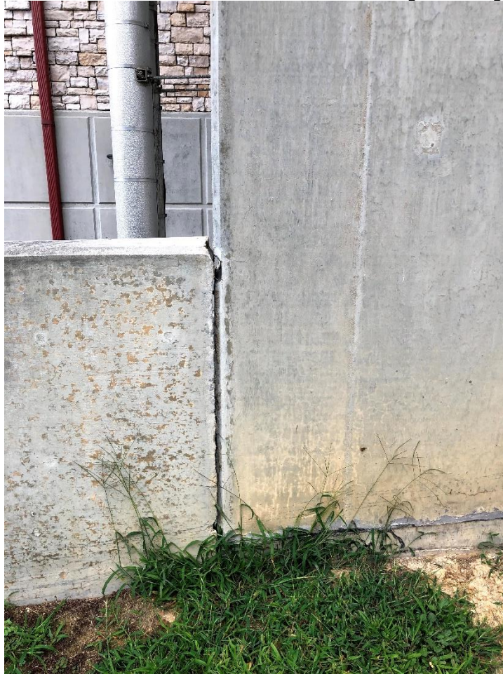
Figure 5.97 – Vertical Crack in Administration Building Retaining Wall
