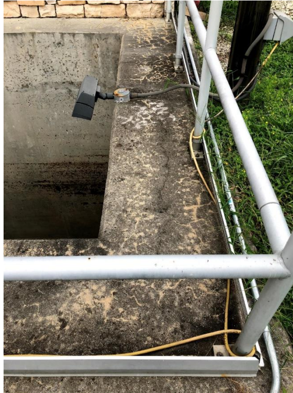
Figure 5.32 – Alligator Cracking Pattern at Top of Wet Well Wall
