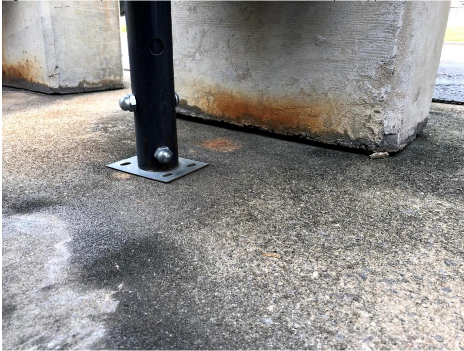
Figure 5.55 – Separation of Aeration Header Concrete Pipe Support from Slab
