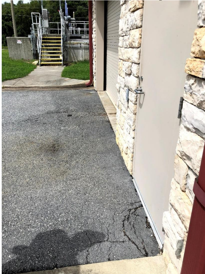
Figure 5.98 – Sinkhole at Utility Building Door
