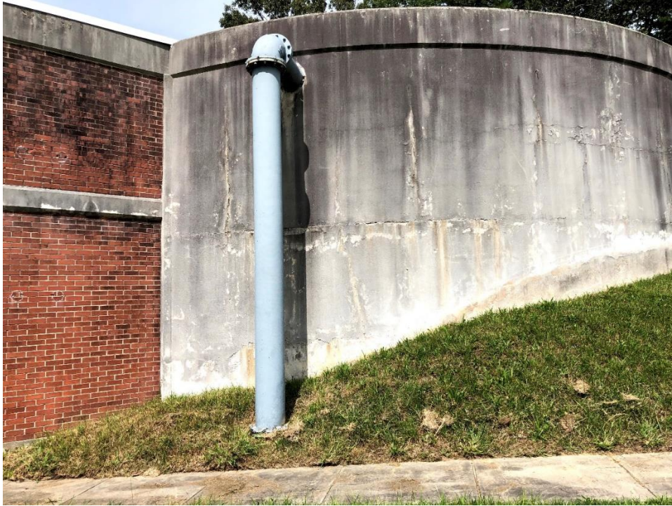
Figure 5.85 – Gravity Thickener #1 Vertical and Horizontal Cracks at Front
