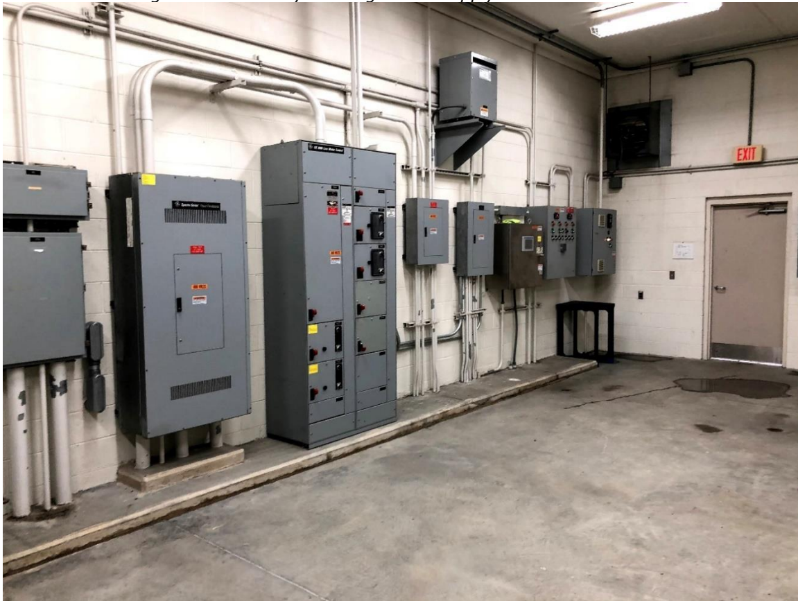
Figure 5.73 – Utility Building Power Supply and Control Panels
