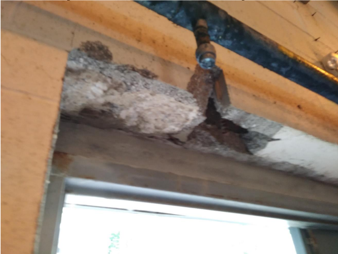
Figure 5.95 – Belt Filter Press Room CMU Lintel Degradation
