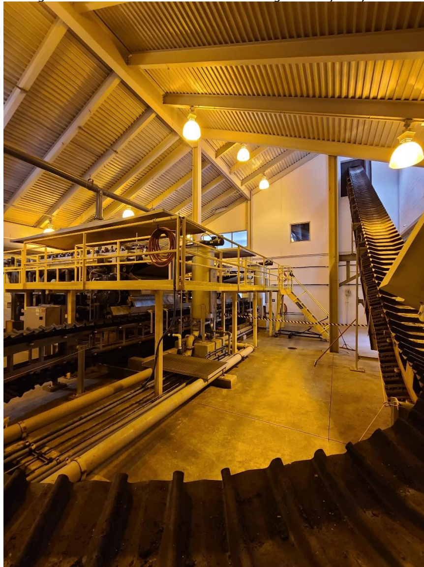
Figure 5.90 – Belt Filter Presses and Sludge Conveyor System
