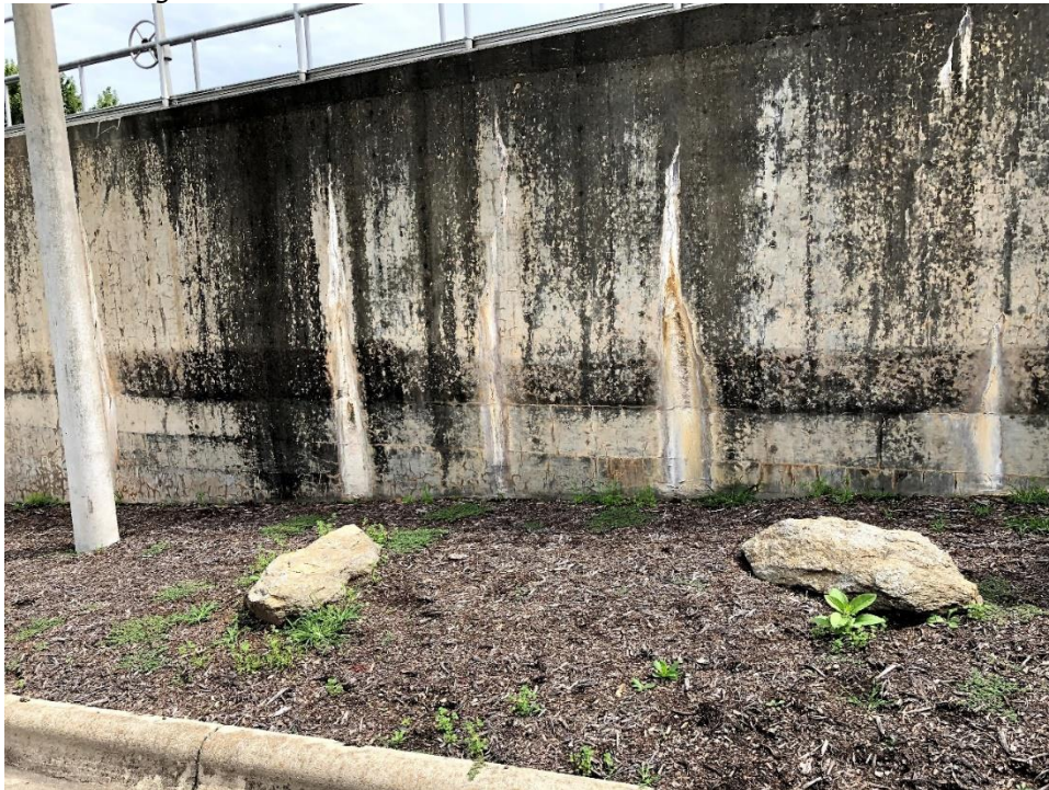
Figure 5.45 – Aeration Basins Vertical Cracks on West Wall
