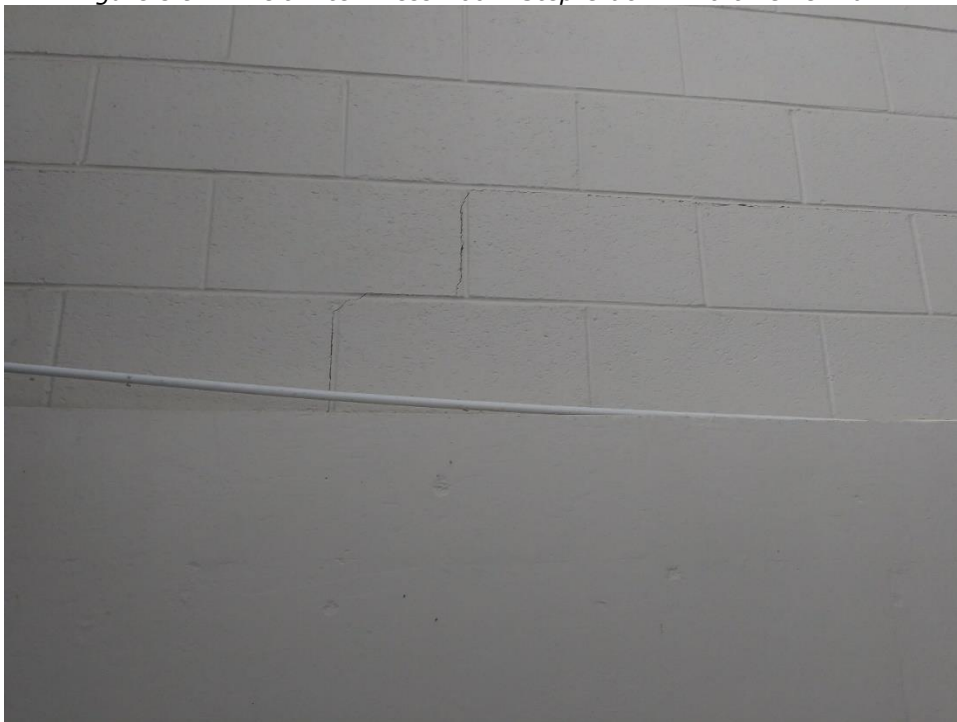
Figure 5.94 – Belt Filter Press Room Step Crack in North CMU Wall
