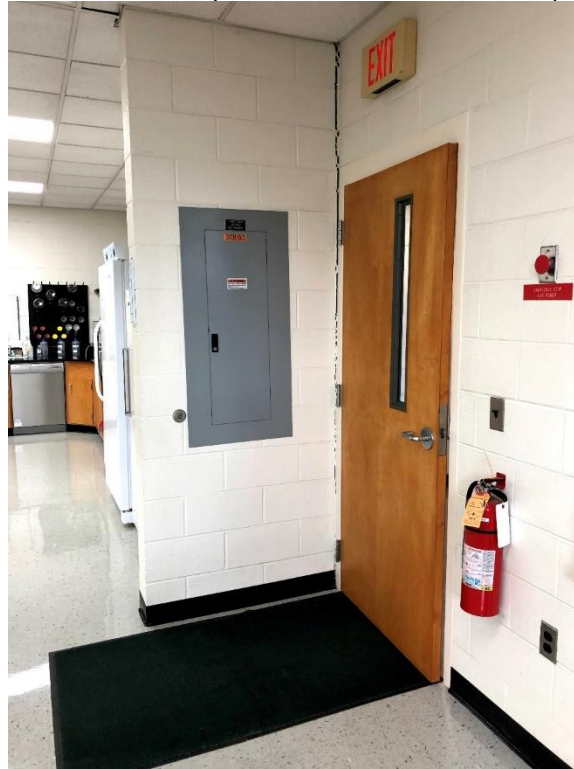
Figure 5.22 – Laboratory Vertical Crack and Wall Separation
