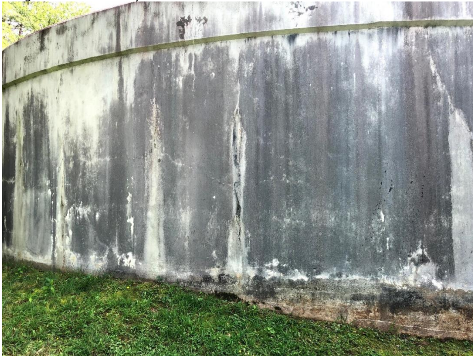
Figure 5.86 – Gravity Thickener #1 Vertical and Horizontal Cracks at Rear
