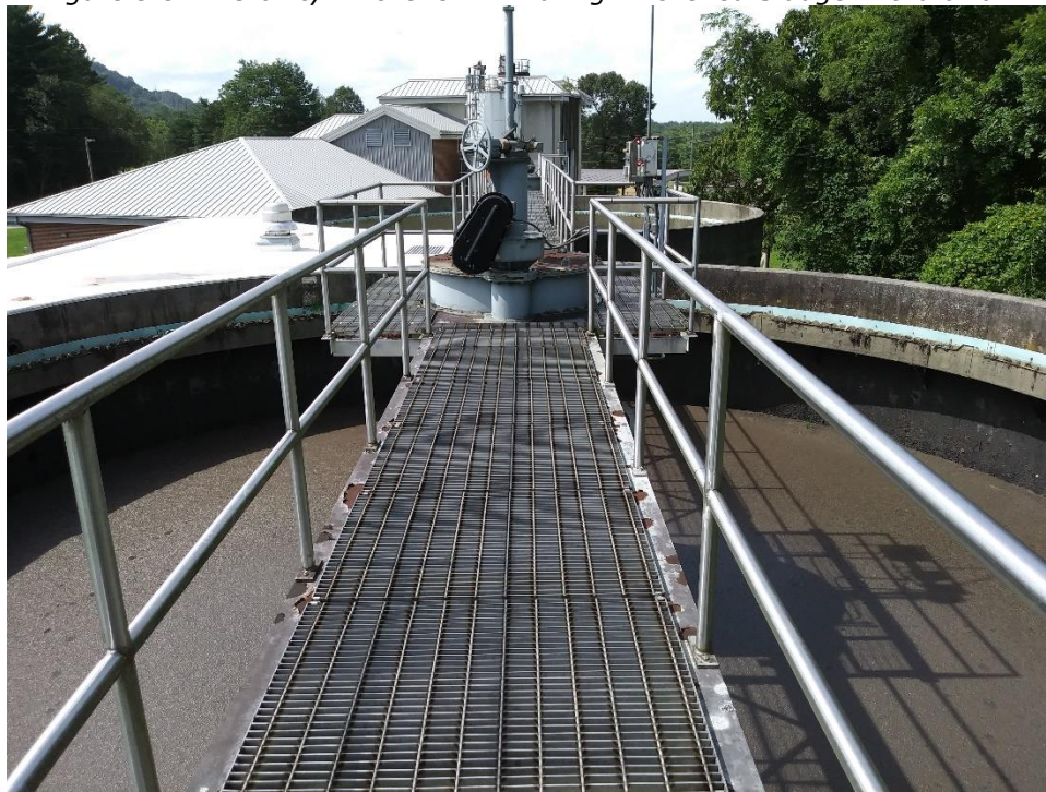
Figure 5.82 – Gravity Thickener #1 During Thickened Sludge Withdrawal
