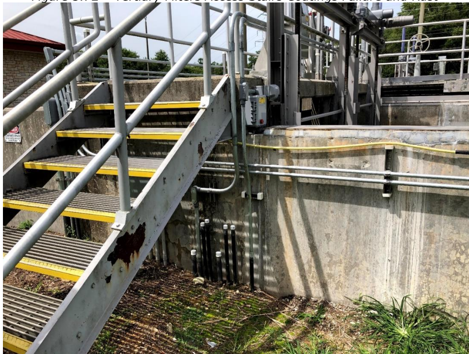
Figure 5.72 – Tertiary Filters Access Stairs Coatings Failure and Rust
