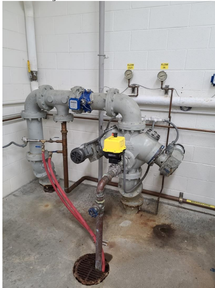
Figure 5.75 – Plant Water Strainer
