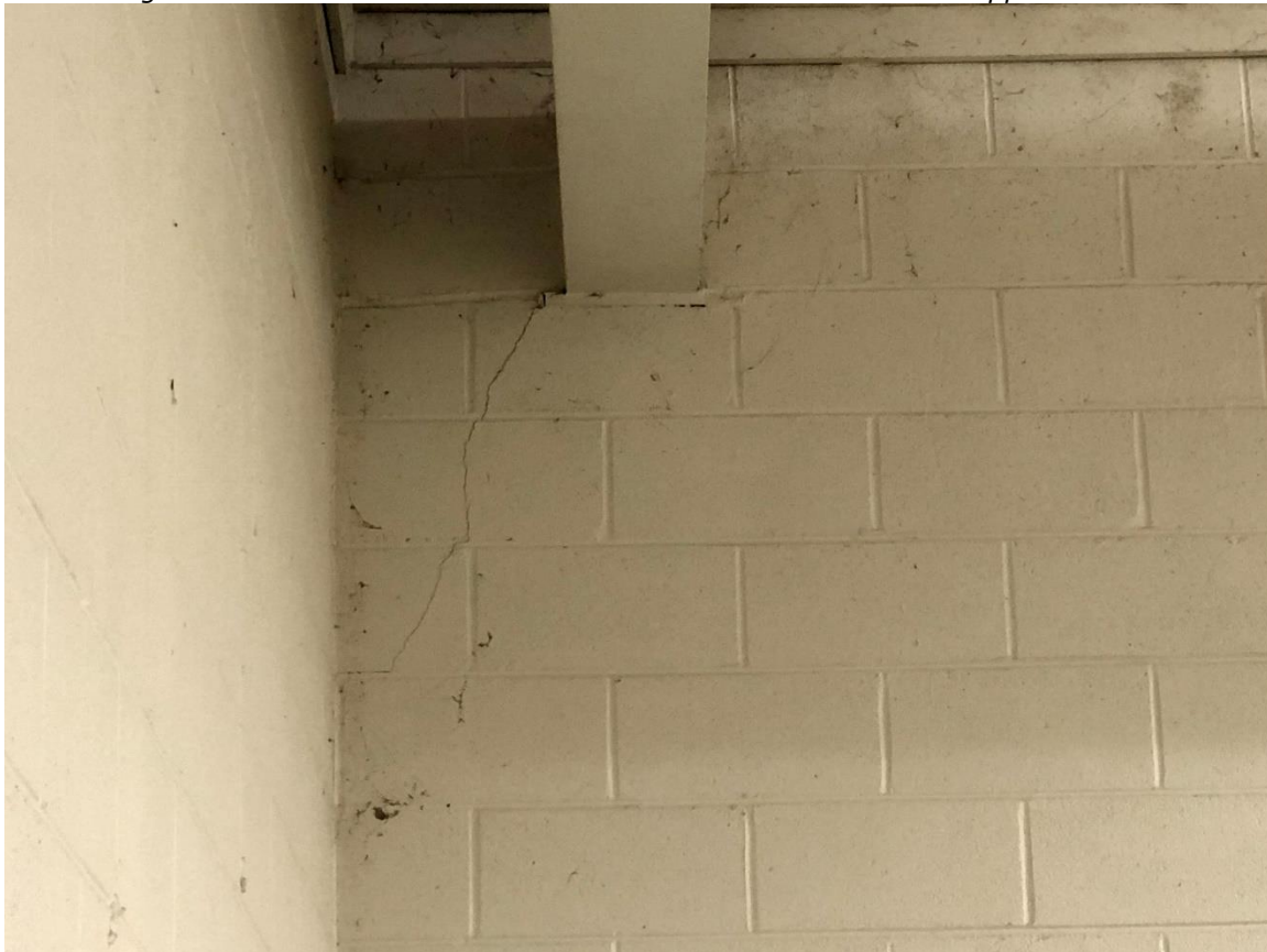
Figure 5.36 – IPS Crack in CMU Wall at Base of Monorail Steel Support Beam
