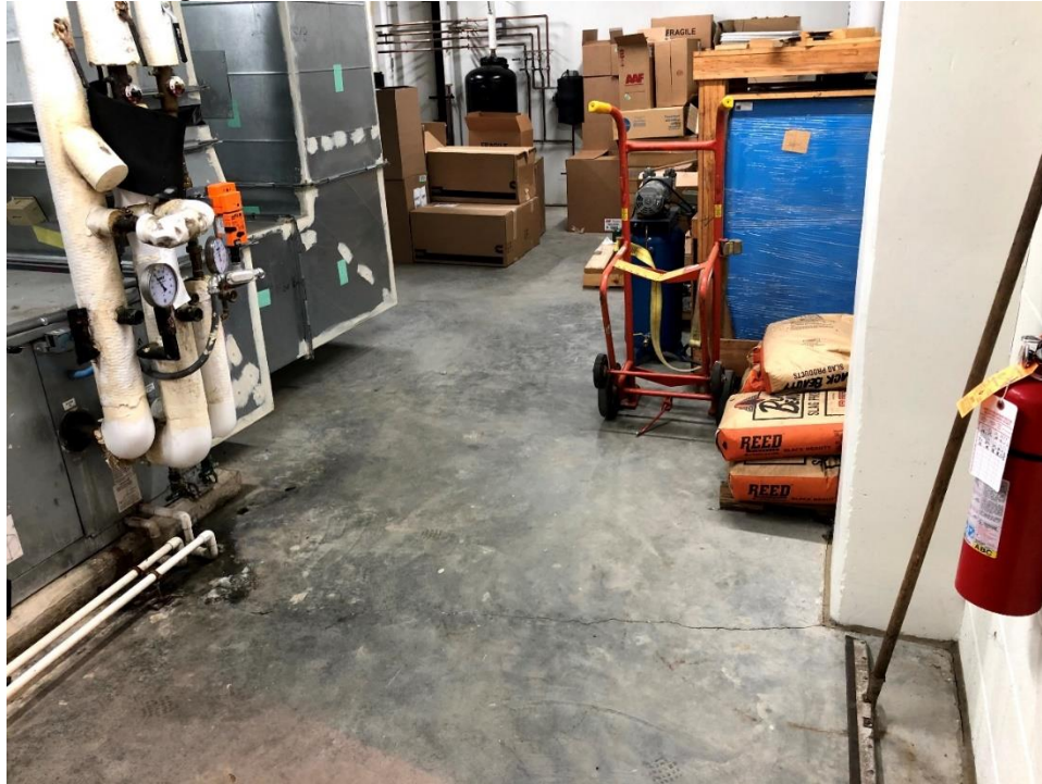
Figure 5.1 – Mechanical Room Cracks in Slab-on-Grade
