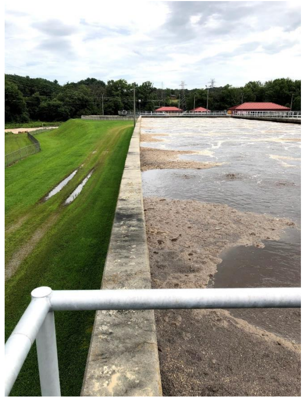
Figure 5.47 – Bow Deflection in Aeration Basin #2 North Wall
