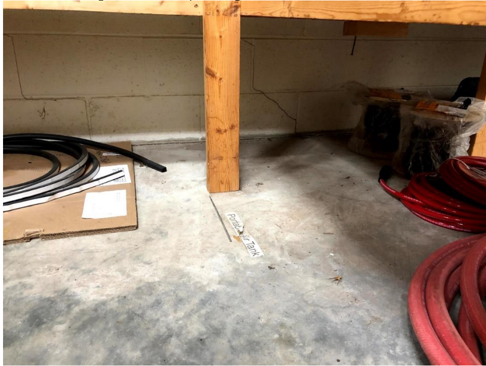
Figure 5.7 – Shop Storage Area Crack in CMU Wall
