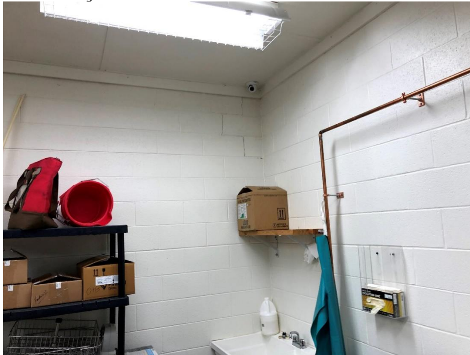
Figure 5.12 – Pretreatment Room Cracks in CMU Wall
