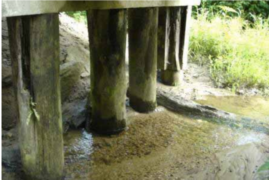
Timber Pile Deterioration
