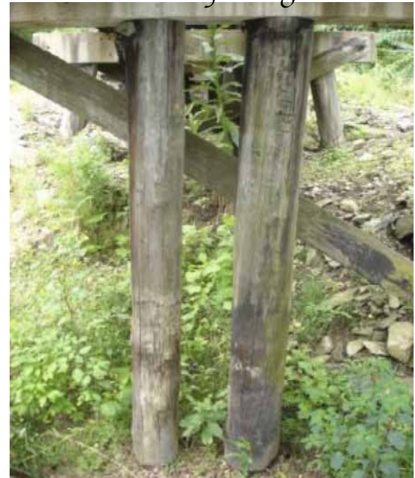
Timber Piles Deflecting
