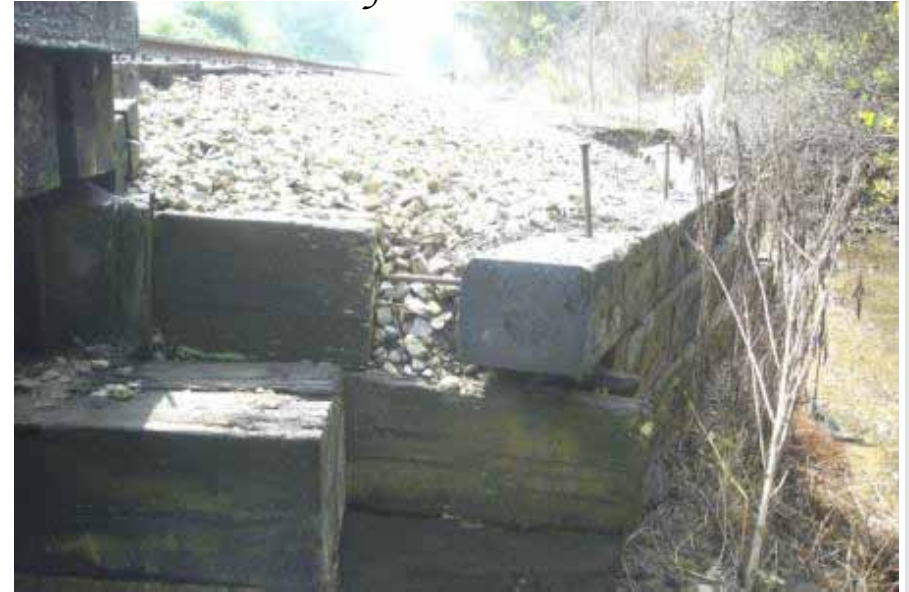
South Back Wall Deflection
