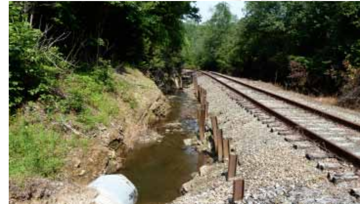
There are some areas with erosion or other environmental degradation along the rail line that may require remediation.
