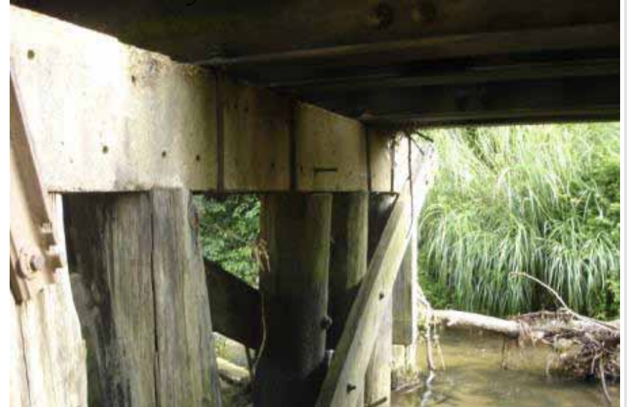
Deterioration of Timber Piles
