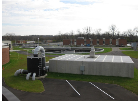
Figure 4. 15,000 SCFM Biofiltration Unit, Middletown, Ohio
