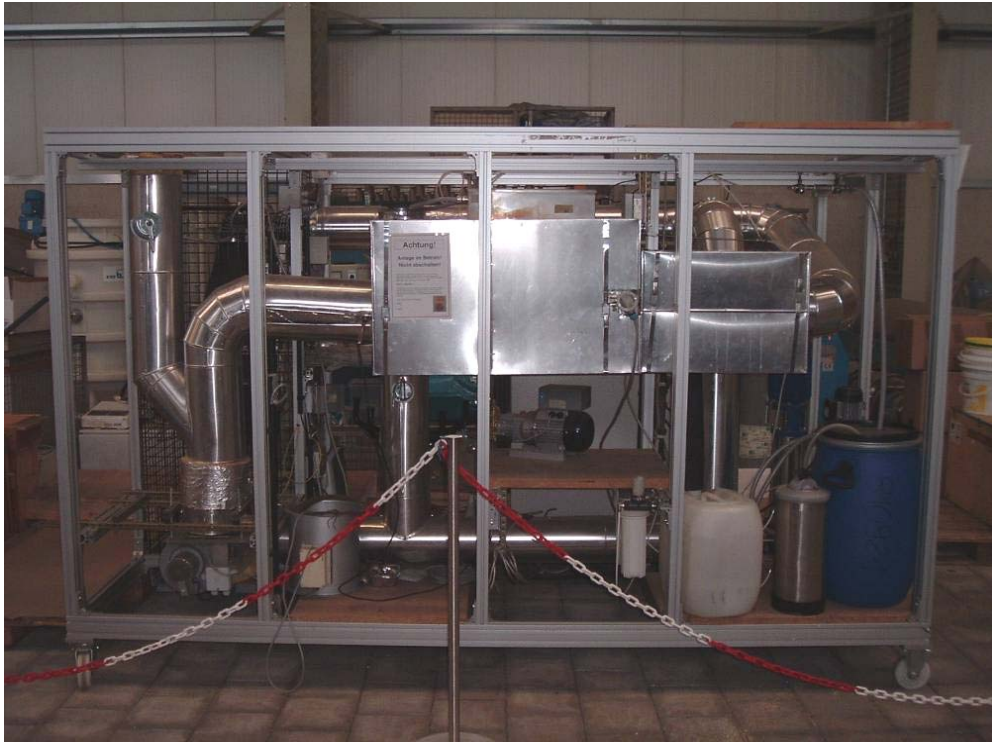
Figure 2: Pilot dryer for simulating belt drying of extruded sludge
